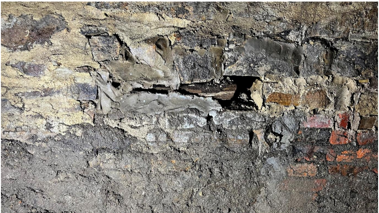
End of flue in boiler room.
